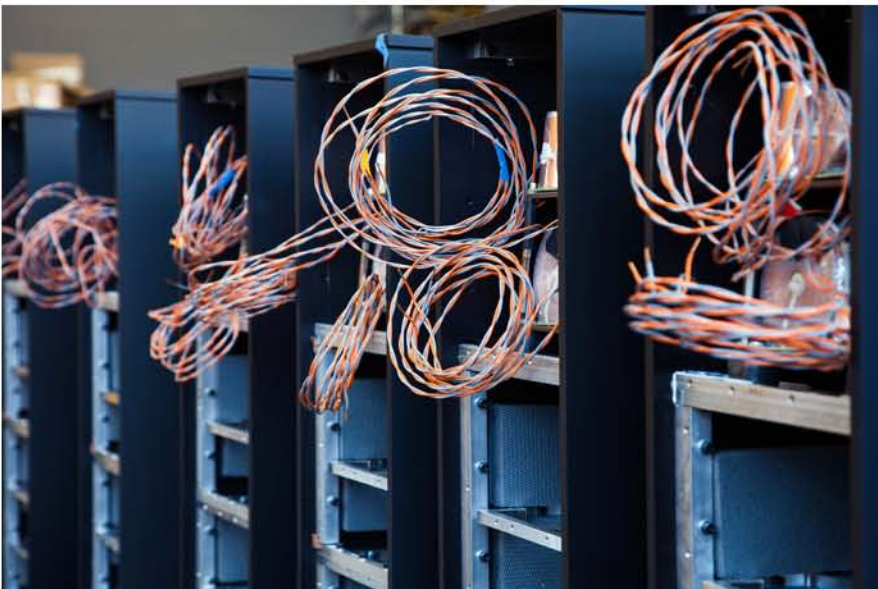
Finished crossovers are housed in dedicated compartments within the Q-series enclosures
